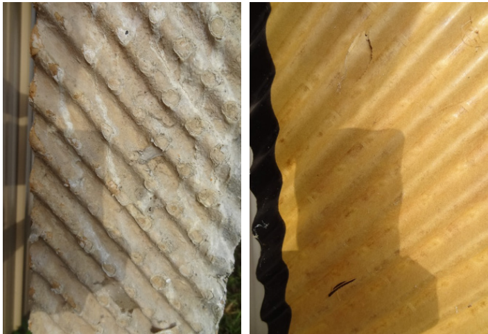
Figure 5. While the front of the pad may look clean, the flutes within the pad can be much dirtier resulting in air restriction that people may not be aware is there.
